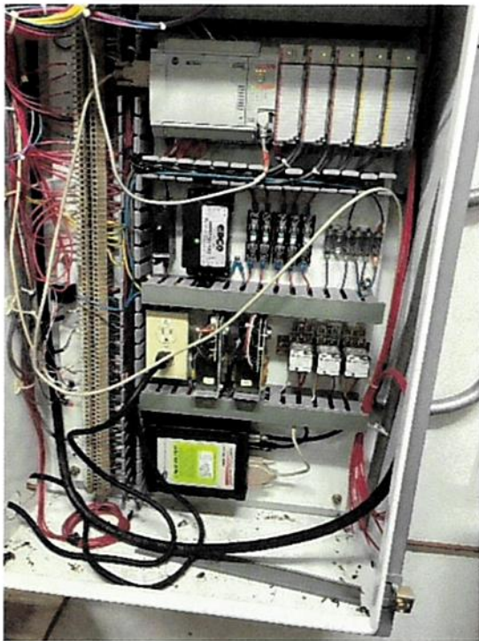
Photo 5 West Water Tower & Well 5 PLC is Discontinued
